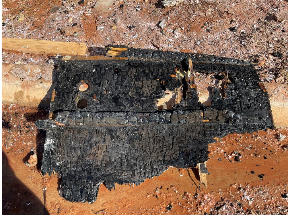
Bottom of flooring from 4 th floor electrical room; southwest area of building
