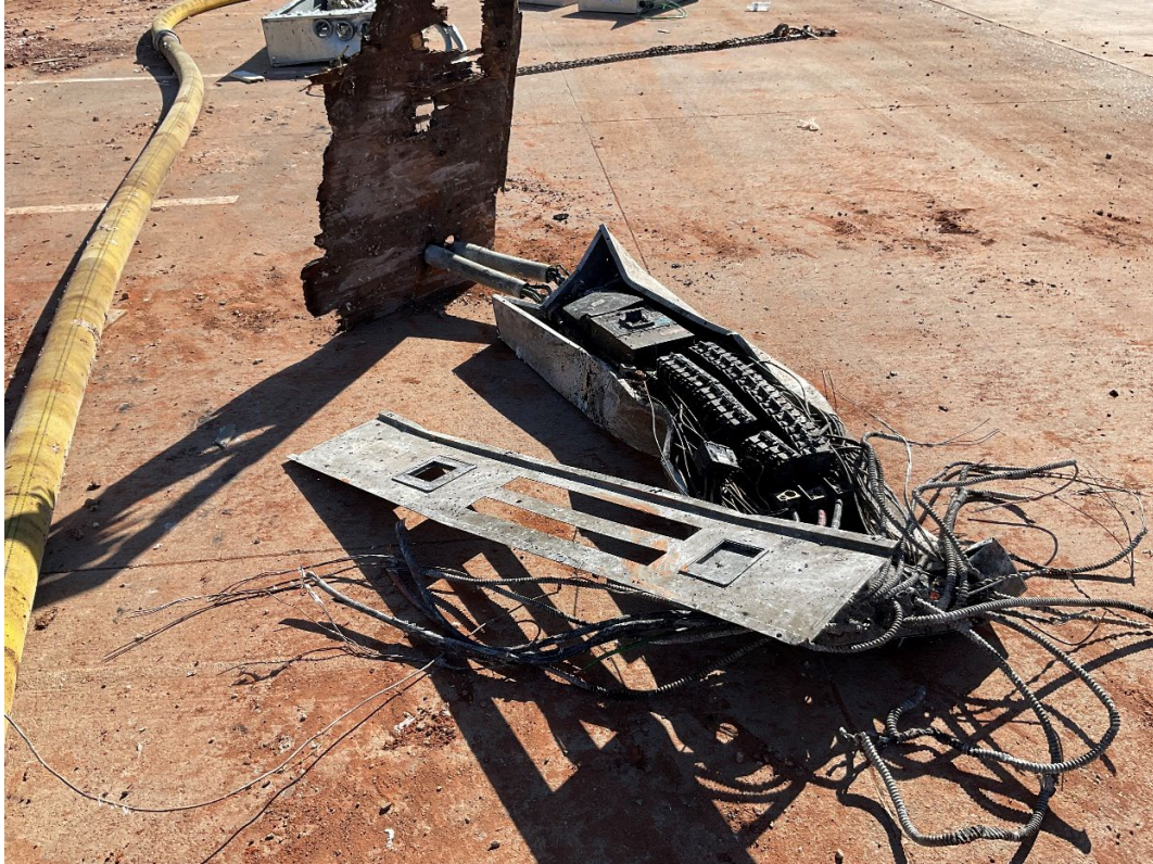
4 th floor sub-panel and a piece of flooring
